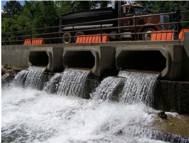
Gavilan Canyon Road bridge over Rio Ruidoso, showing fish barrier and scour pool
