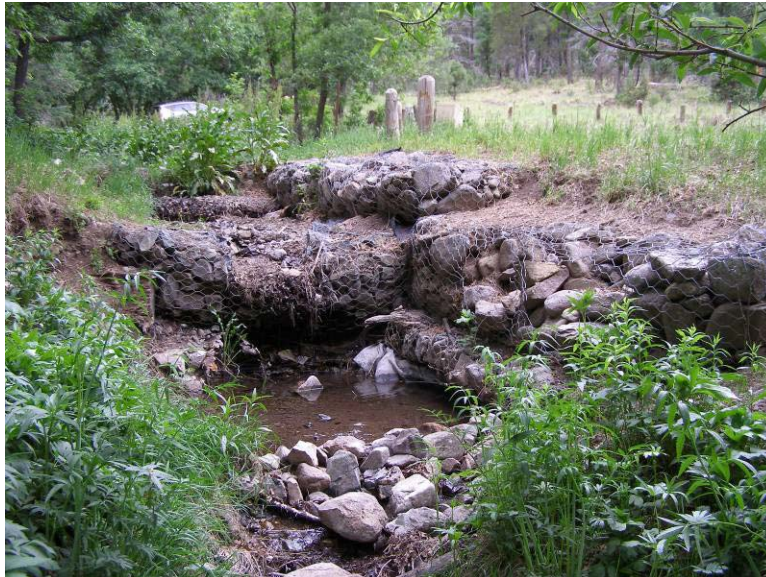
Undercut Gabion revetment on Eagle Creek
